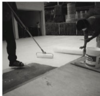
Lay the next roll of fabric so it overlaps the edge of the prev. row 2.5 – 3". Continue laying Rows of fabric until the whole surface is covered.
