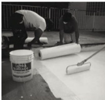
When you reach of the end of the deck cut the fabric with scissors or knife and start laying the next row.
